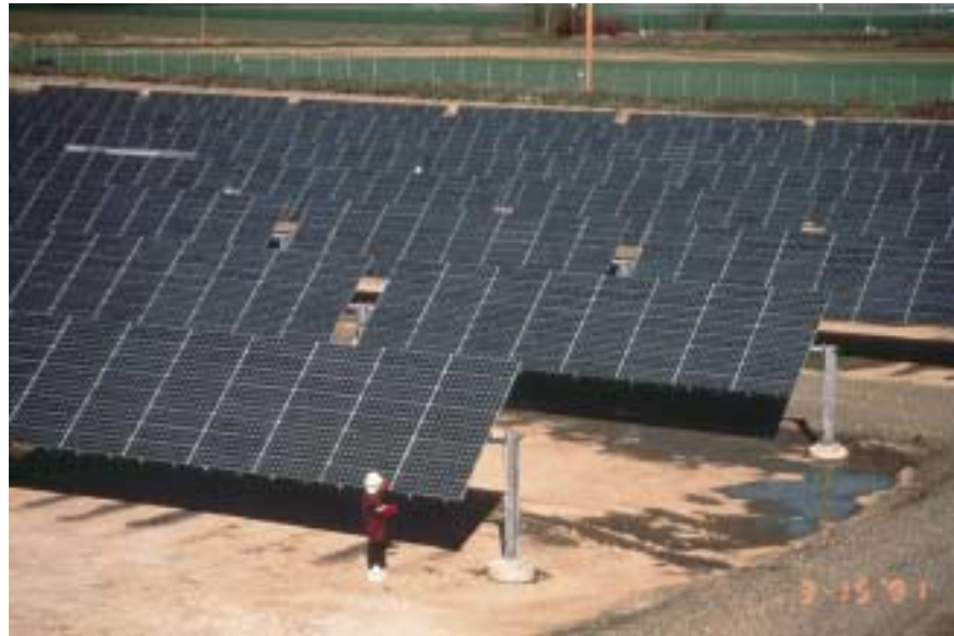
FIGURE 2–19 Solar panels. Davis California Pacific Gas & Electric PVUSA (Photovoltaic for Utility Scale Applications). Solar panels produce dc which must be converted to ac before being fed into the ac system. This plant is rated at 174 kilowatts. (Courtesy Siemens Solar Industries, Camarillo, California)
