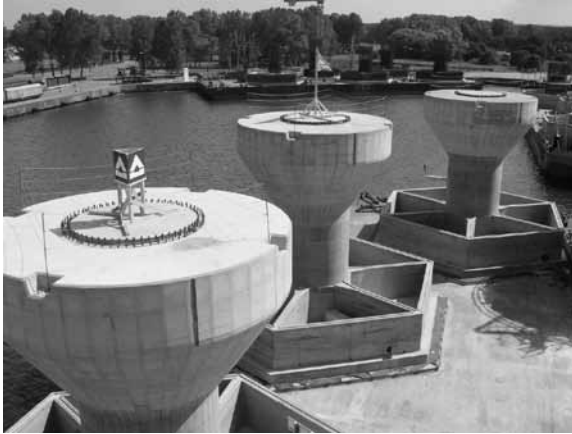
16.4 Fabrication of concrete gravity based foundations, for the Lillgrund wind farm, on special barges (© HOCHTIEF Construction AG, Civil Engineering and Marine Works, Hamburg, Germany).
