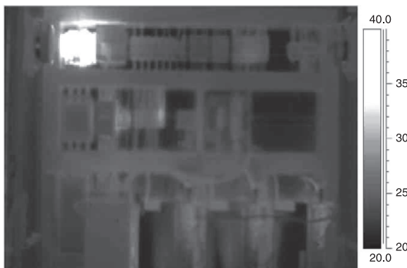
11.6 Thermo image of an electrical cabinet.
