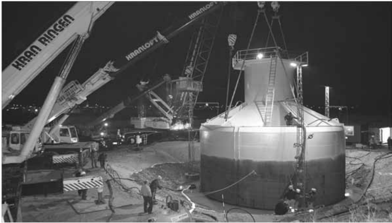
16.11 Prototype of a suction bucket foundation for a 3 MW offshore wind turbine in Frederikshavn (DK) (Ibsen, 2008).
